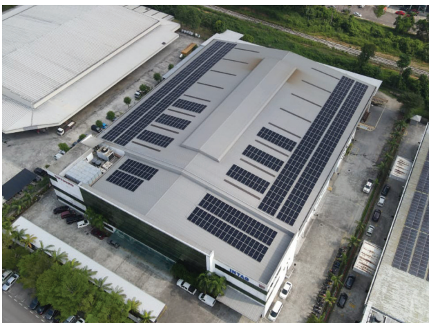
Solar PV system at MTAG Group
