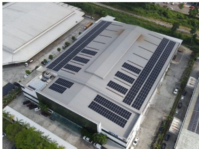
Solar PV system at MTAG Group
