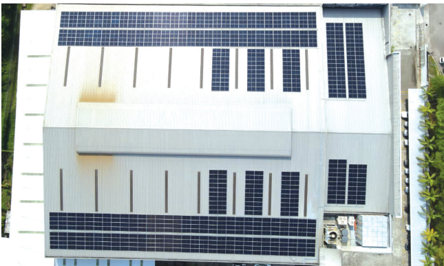
Solar panels at MTAG
