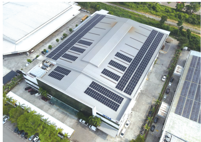
Solar PV system at MTAG
